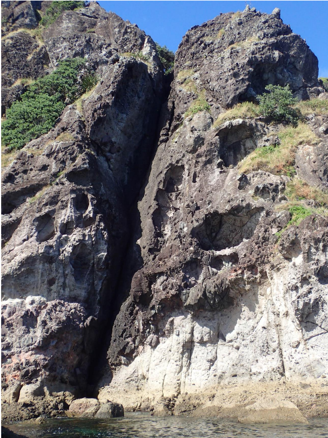
Deep gut eroded along fracture.
