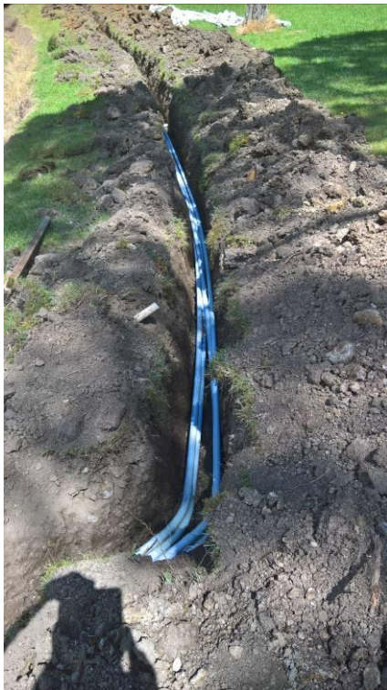
Underground conduit from panels to battery storage under the lodge
